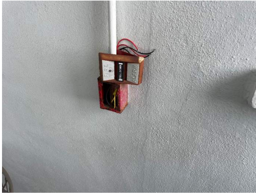
Figure 17: Disconnected fire alarm system.
