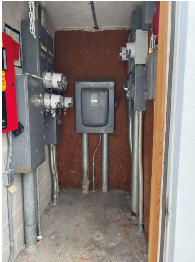
Figure 15: Typical mechanical room overview.
