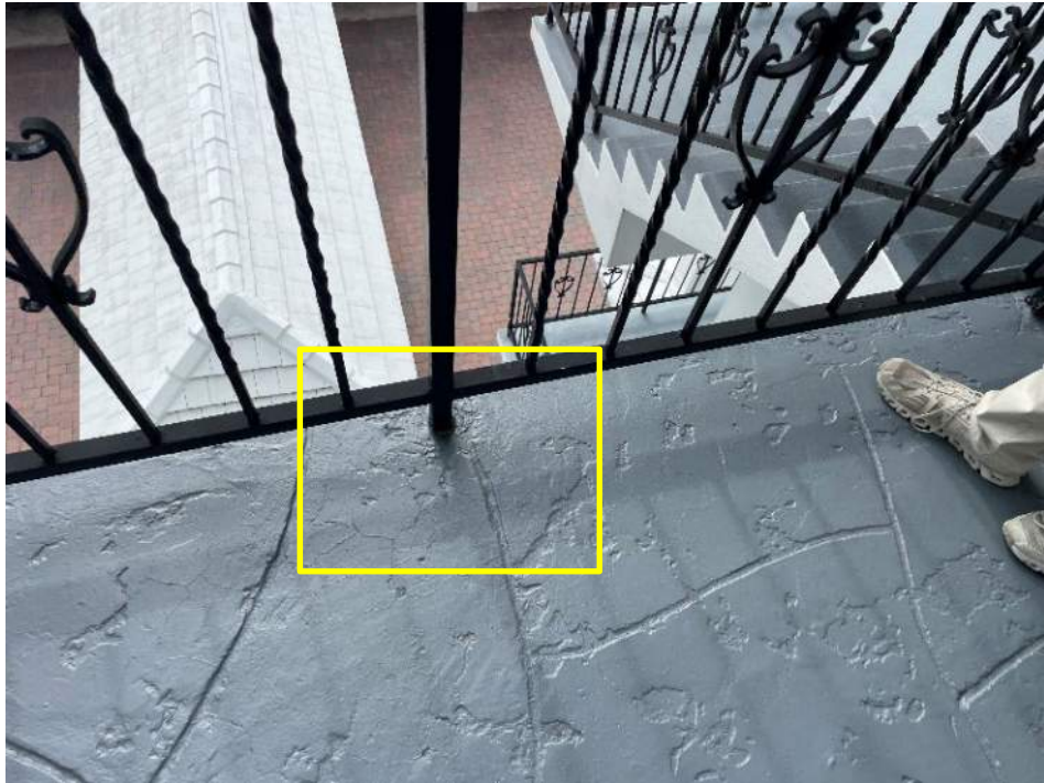
Figure 6: Possible delamination of 3 rd floor balcony at post pocket.
