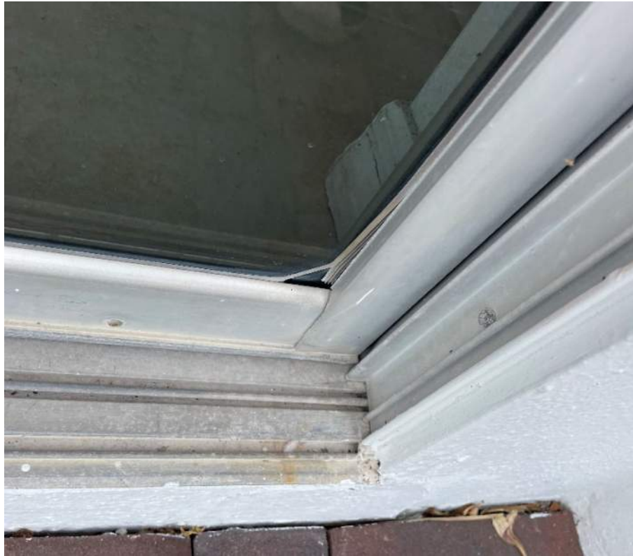
Figure 4 – Glazing pulling apart on sliding door.
