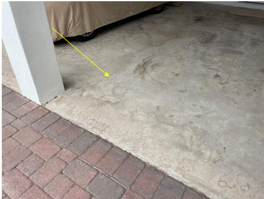
Figure 10 Existing condition of Slab-on-Grade with some nonstructural cracking
