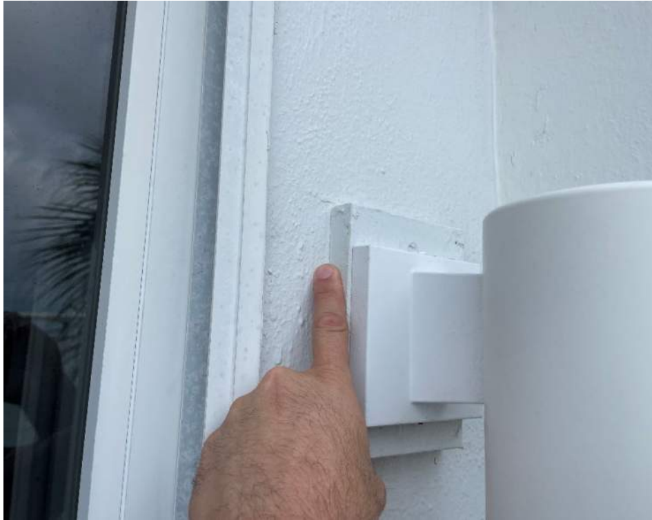
Figure 2 – Missing sealant at ground floor light fixtures.
