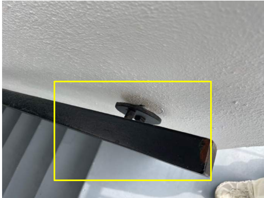
Figure 16: Typical Loose railing connection near stairwell
